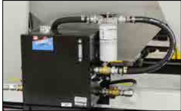
Fig 57 - Hydraulic system and filter
